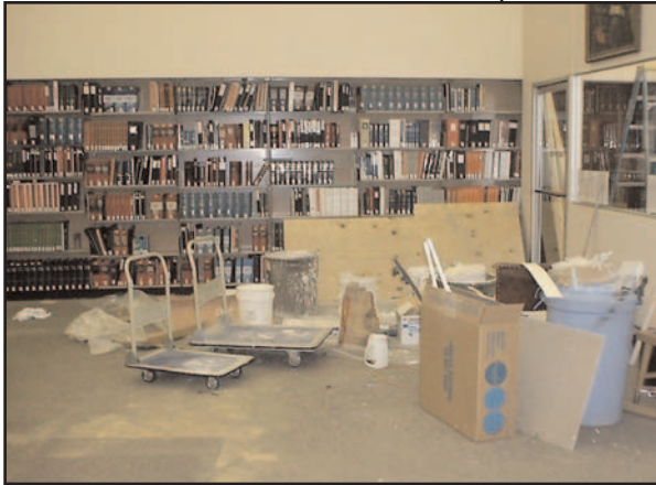
During the remodel, additional patron PCs were installed in the first-floor reading room.
